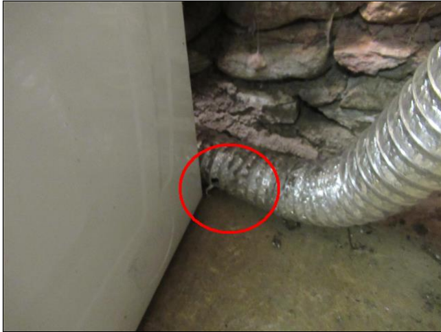
3.15 Item 1(Picture) hole in tje duct
