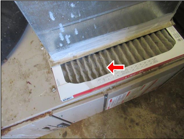
9.3 Item 1(Picture) dirty air filter
