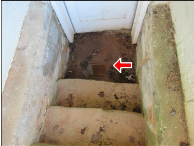
2.4 Item 1(Picture) standing water
