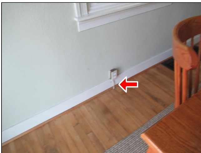
4.6.A Item 1(Picture) protect the wiring
