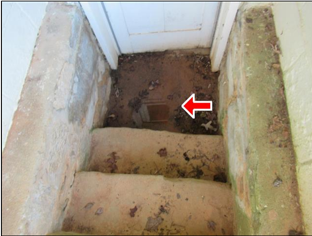
2.4 Item 1(Picture) standing water
