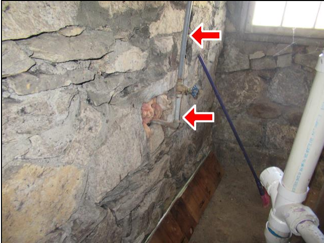
7.1 Item 1(Picture) galvanized and polybutylene
