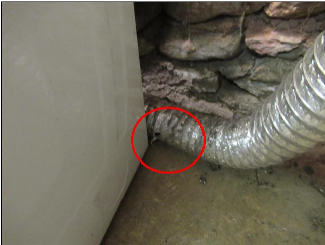
3.15 Item 1(Picture) hole in the duct
