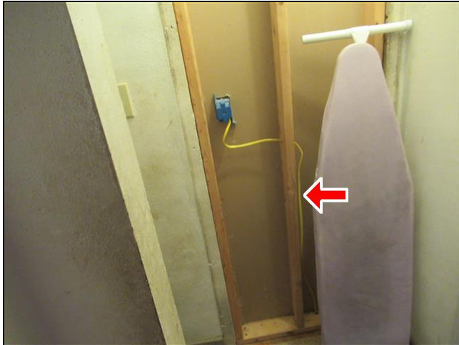
4.6.B Item 1(Picture) protect the wiring
