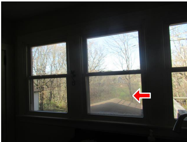
3.4 Item 1(Picture) kitchen window
