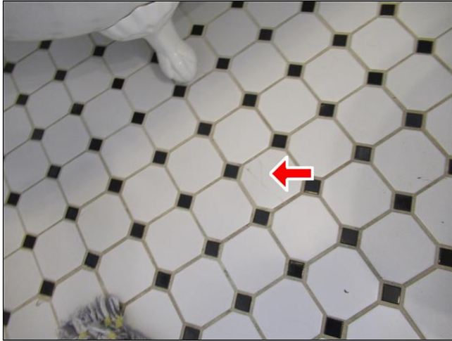
5.7 Item 1(Picture) cracked tile
