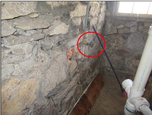
7.3 Item 1(Picture) main water shut off valve
