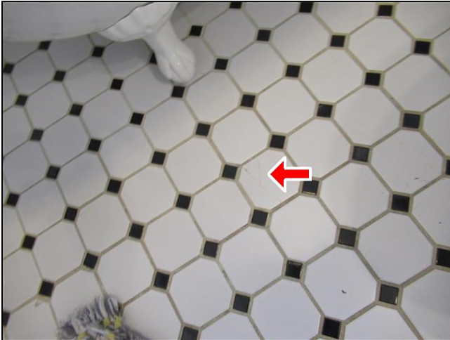
5.7 Item 1(Picture) cracked tile
