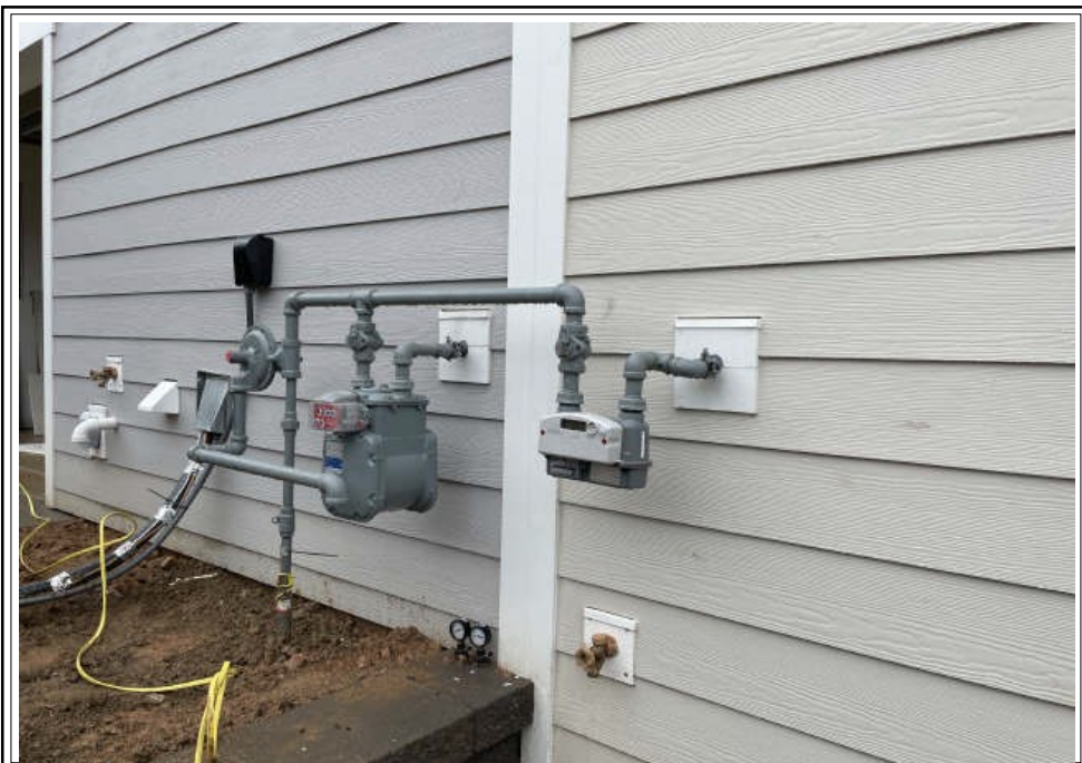
Utilities not connected
